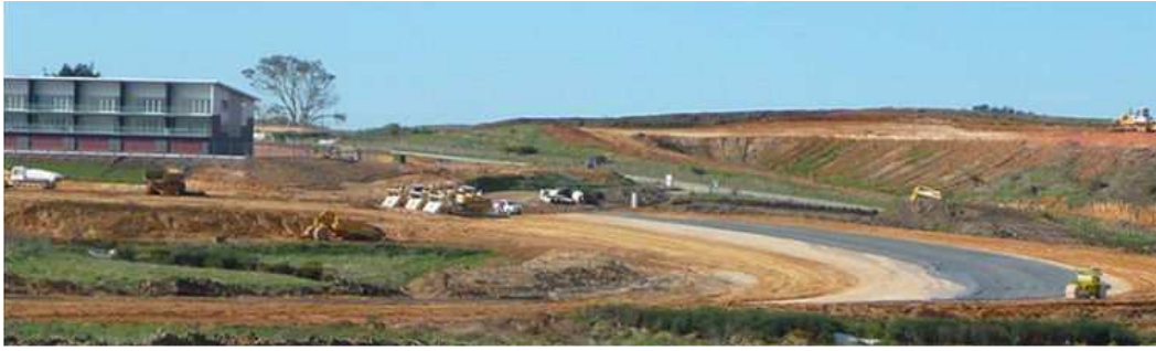
Turn 1 has now been formed and a layer of gavel has been laid and rolled.
